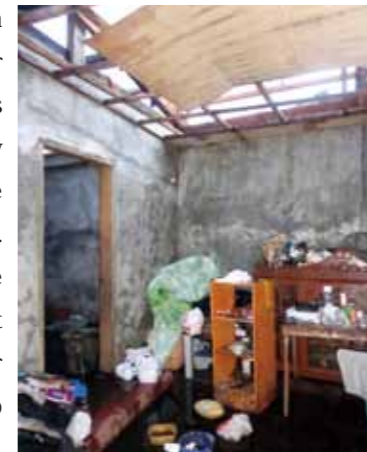
(a) Exposed ceiling beams and destroyed roof structure
