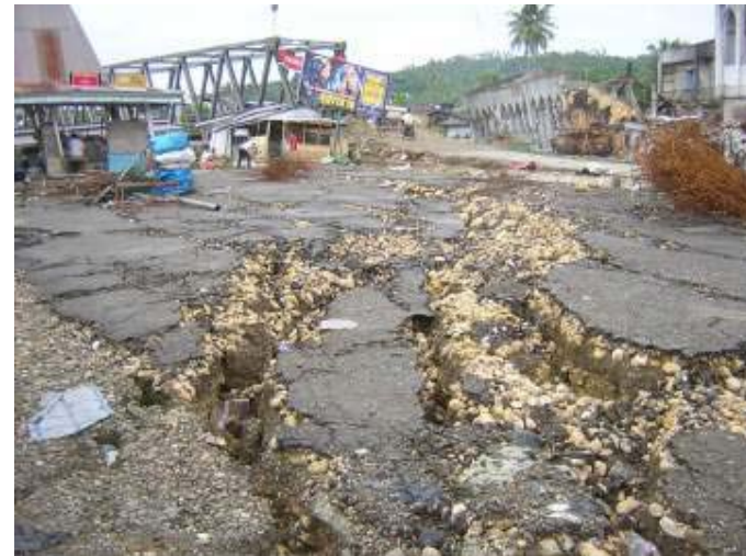
Liquefaction Damages in Gunung Sitoli
