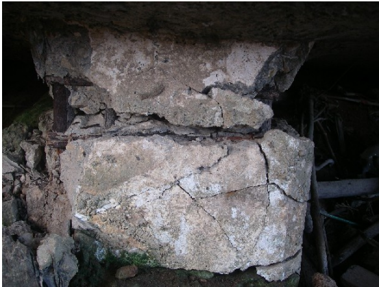
(c) Broken cast-in pile head (NW-Ab.)
