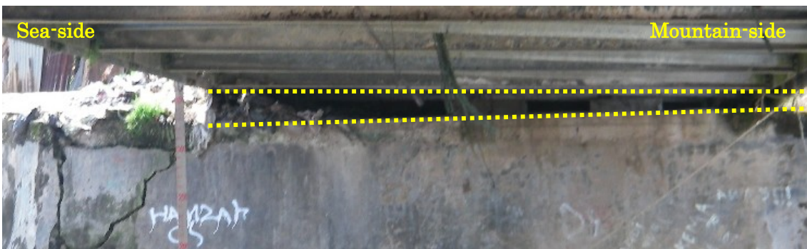
(e) Uneven settlement of the SE abutment. The settlement at the seaside of the pier is greater than that at the mountainside
